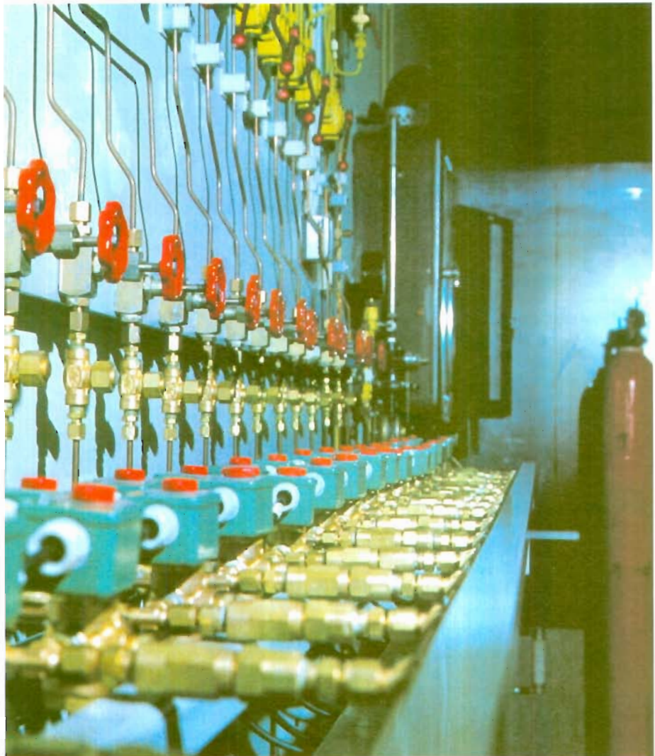
A valve system specially designed and built at the Gasinstituut for the gas mixing station, controls the movement of different gases from the station into the laboratories for testing and analysis.
